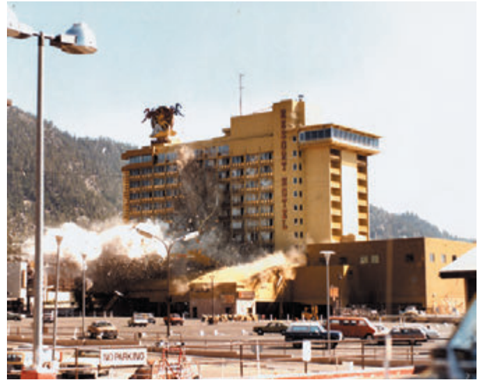
DTRA's force protection experts analyze the effects of explosives on building structures.
