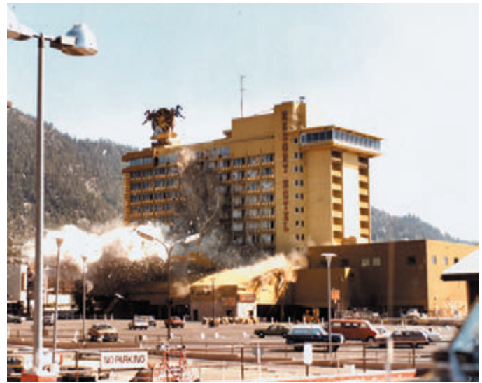
DTRA's force protection experts analyze the effects of explosives on building structures.
